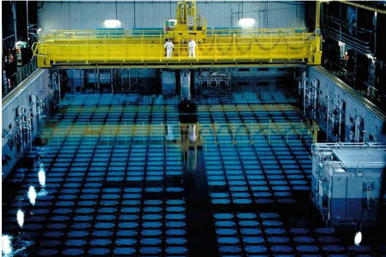
Example basin with spent nuclear fuel under water
